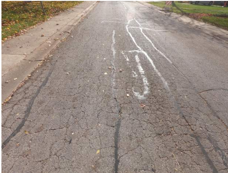
PASER 3 – Mohawk Drive (Burlington Ave to Norfolk Ave)
